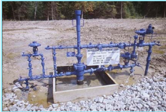
At the wellhead
