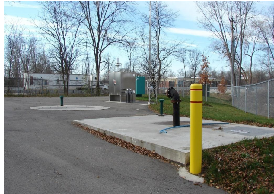
Michelson Pump Station
