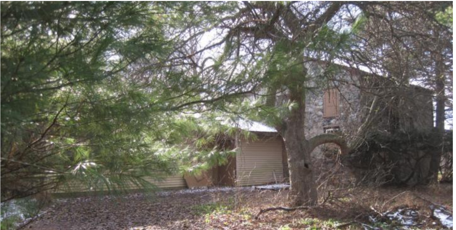
View of the rear (east), addition proposed for removal in the foreground
