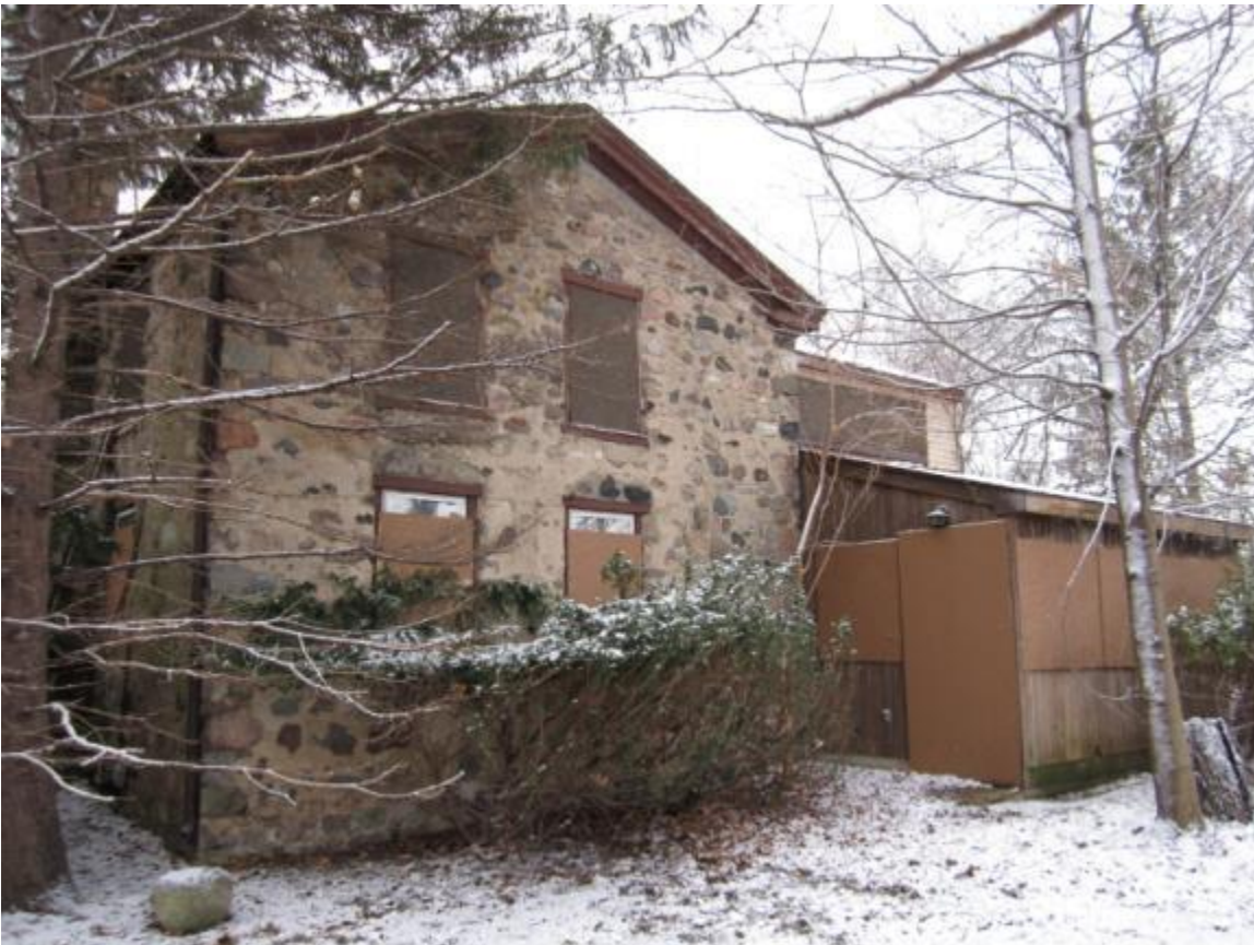
Detail of front (west) elevation, wood sided one-story porch/addition proposed for removal
