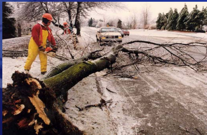
Storm Damage Cleanup
