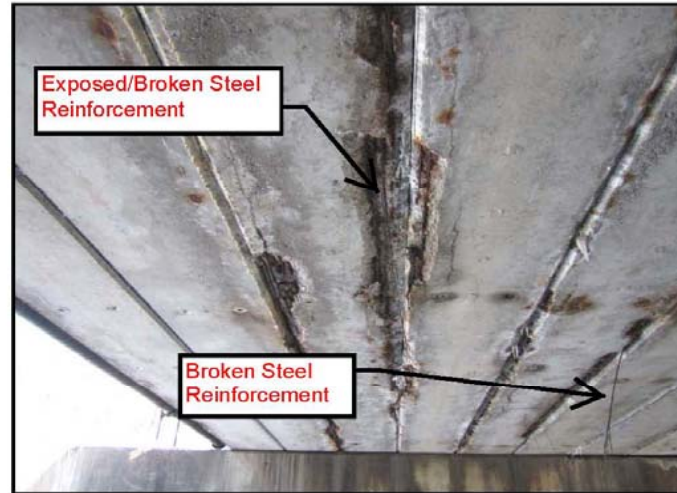
Exposed/ broken strand in northside beams
