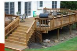
Wood Deck Construction Structural Issues
