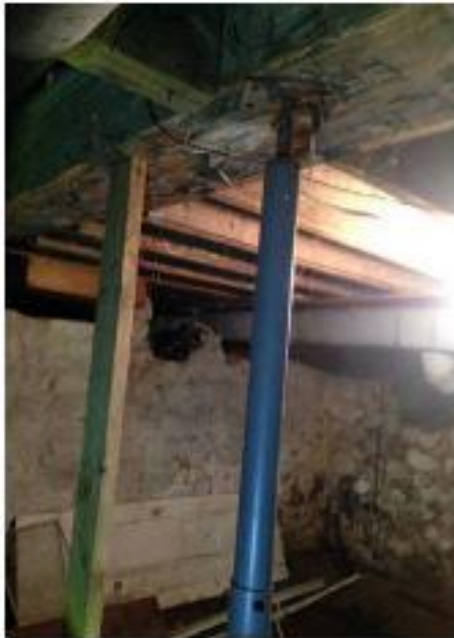
Improper support posts and torque at support beam.
