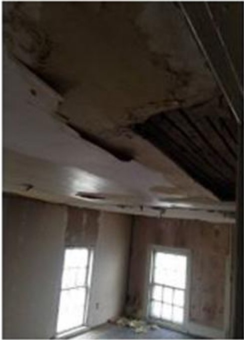
Water damage at ceiling from roof leaks.
