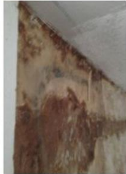
Heavy water damage at second story at rear of home. Mold growth observed.
