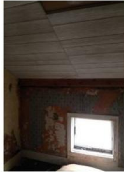
Water damage at ceiling and walls.
