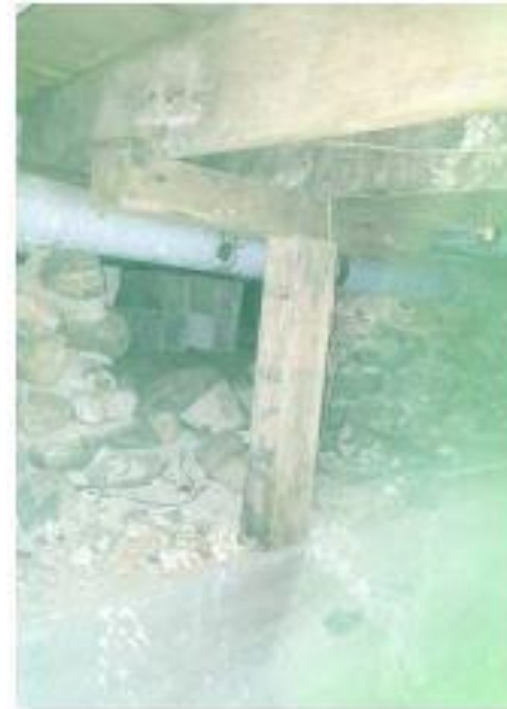
Improper support post at crawlspace.
