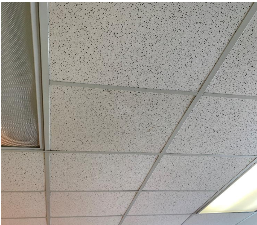
View of 2' X 2' Suspended Ceiling Tile – Pin Holes (HA3)
