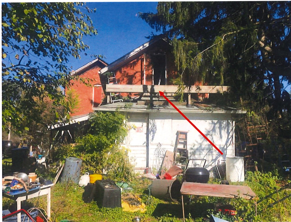
Rear, south side of structure looking north. Note unconventional framing over one-story portion.
