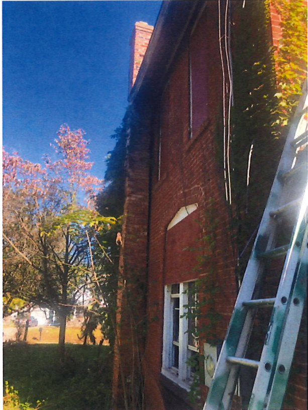
Alternate view of chimney displaced away from structure.
