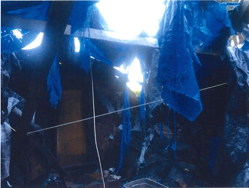
Roof and ceiling framing missing over portion of second floor.
