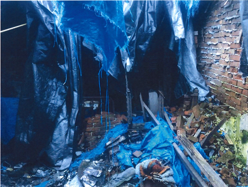
Failed load bearing brick wall at second floor.
