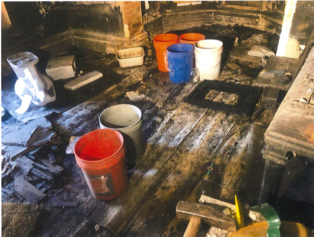
Delaminated flooring at first floor. Note buckets to collect water.
