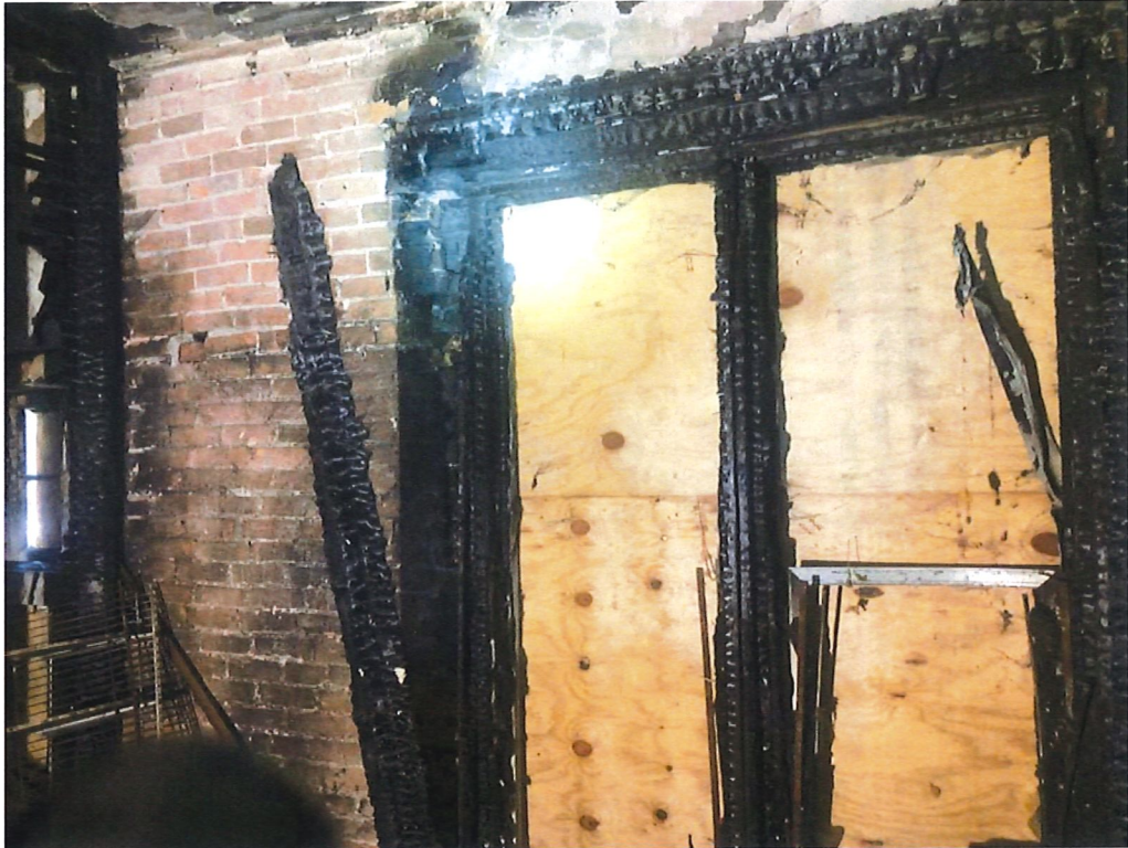
Another example where there were no interior wall studs against the exterior brick.
