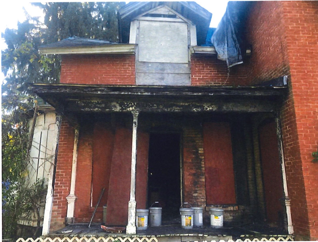
Front porch on north side of structure. Note portion of roof missing behind dormer.
