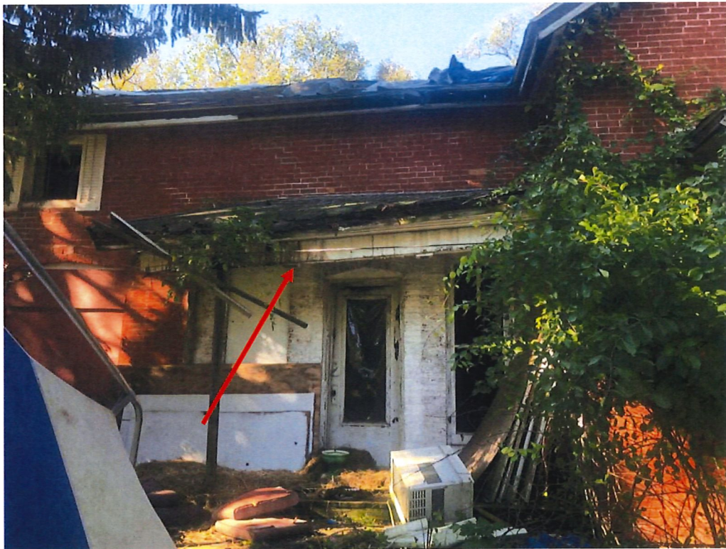
Arrow points to deteriorated roof framing over porch at east entry.
