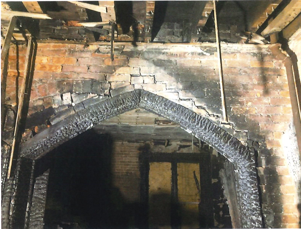
Interior structural brick wall damaged at opening on first floor.
