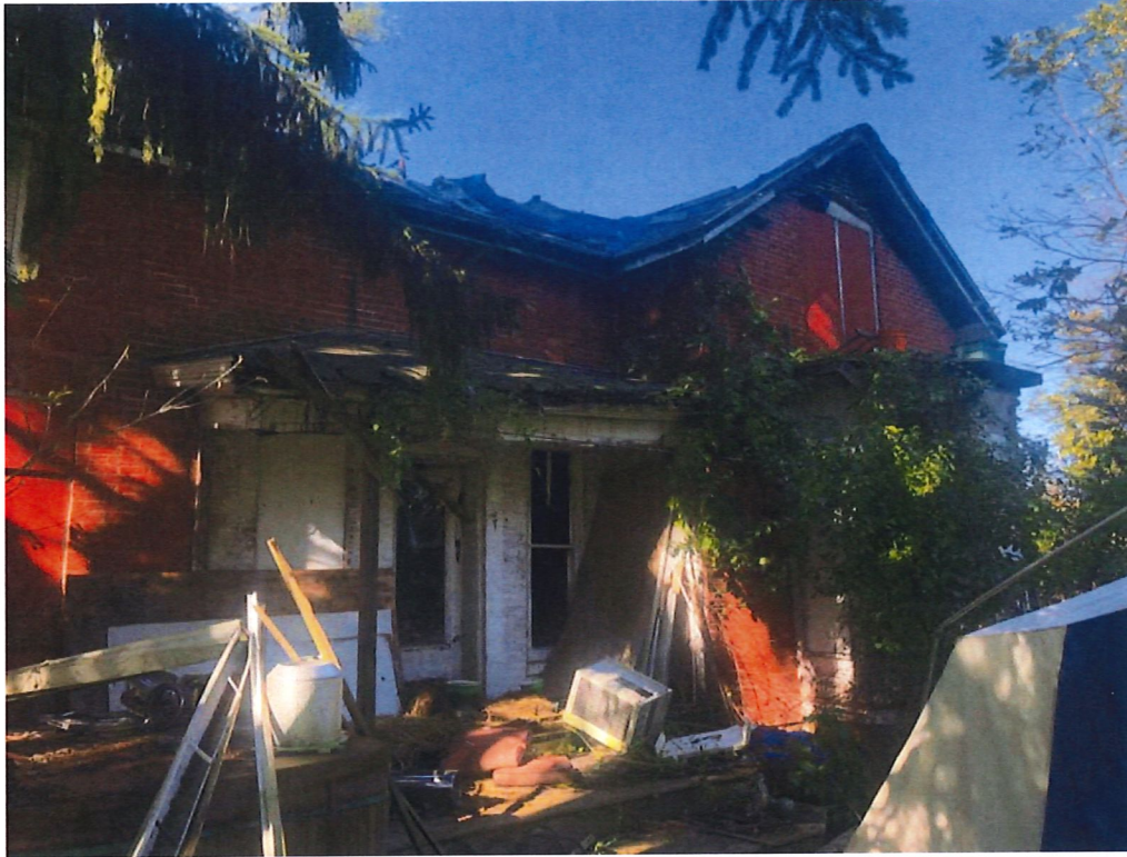
Alternate photograph of east side of structure looking northwest. Note missing roof area.
