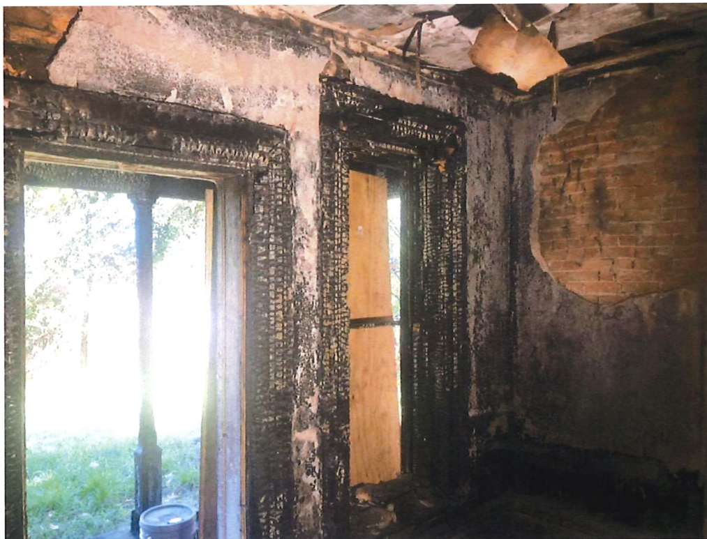
Exterior brick wall. Note that there were no wall studs against the brick.
