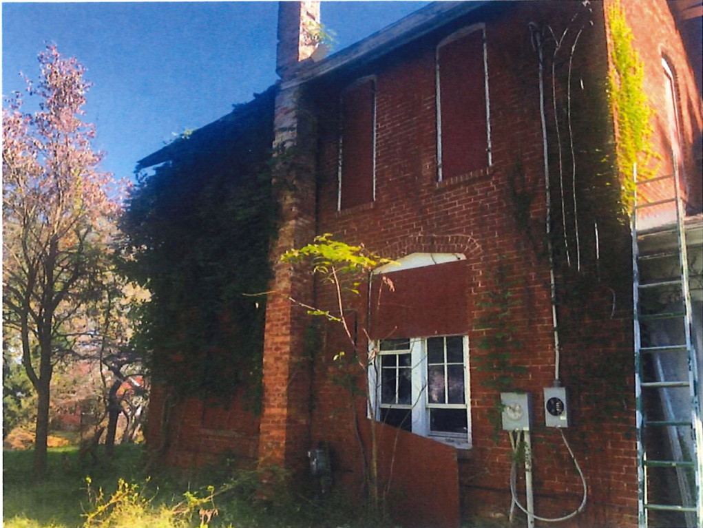
West side of structure looking northeast. Note chimney displaced away from structure.
