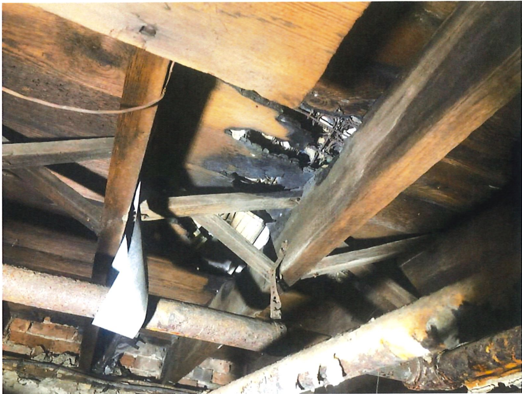
Portion of first floor framing with fire damage.
