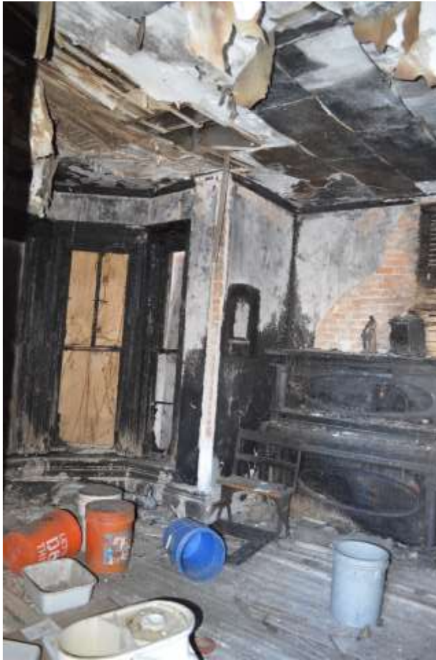
17 – Looking at fire damaged interior, damaged east bay window to left, January 2021
