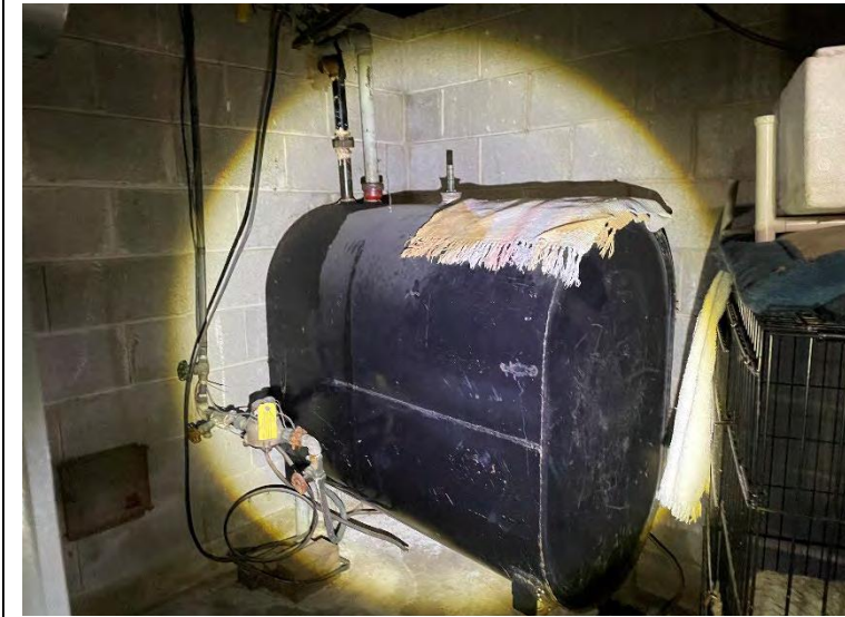
Photo 13. AST in northeast corner of basement
