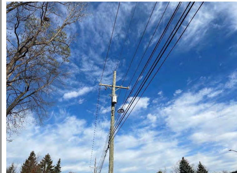
Photo 18. Pole mounted transformer at northeast corner of Subject Property
