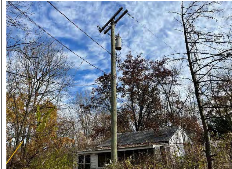
Photo 7. View of post mounted transformer and garage, facing northeast
