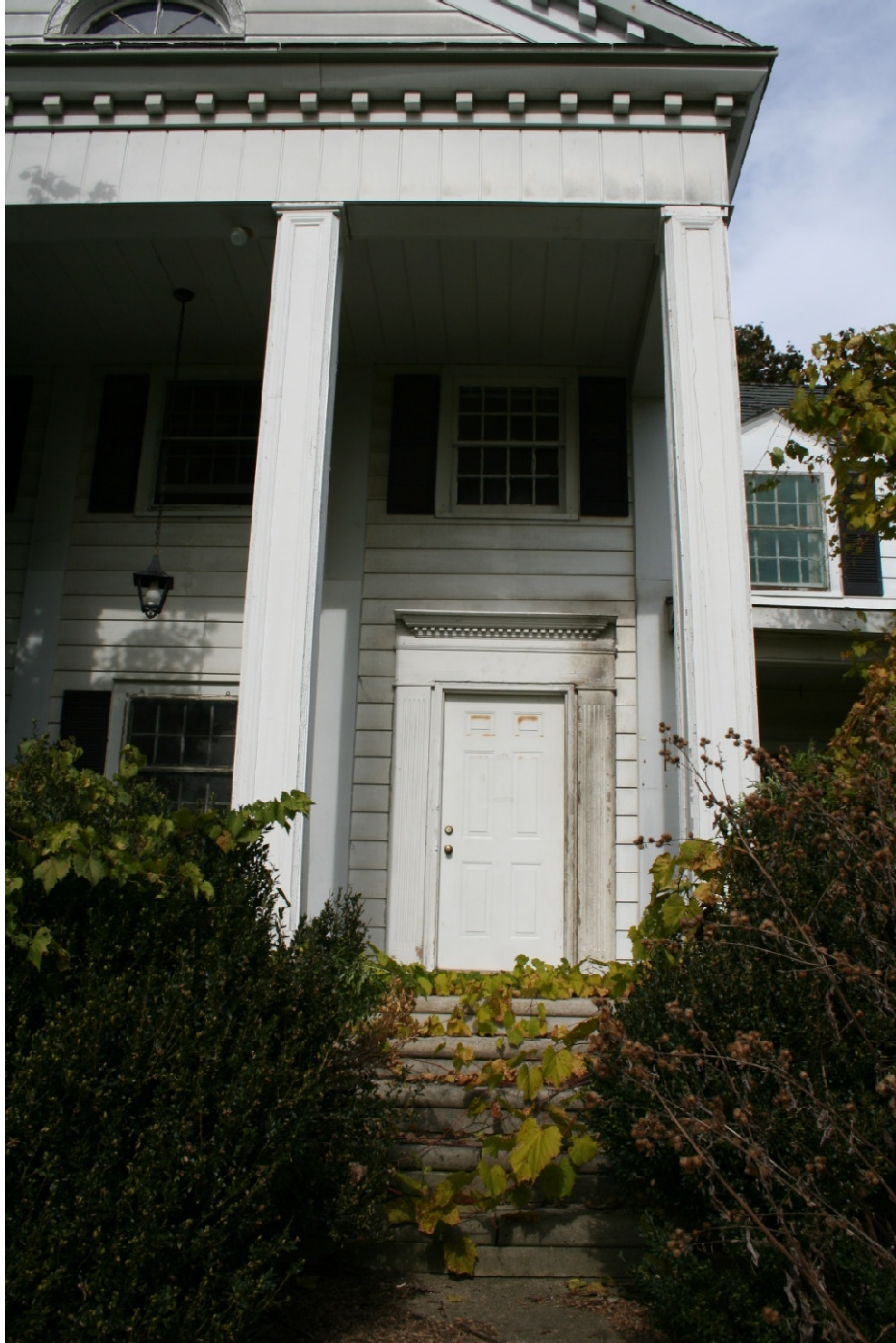
Detail of main entrance looking north, note non-proportional columns and door surround, October, 2009
