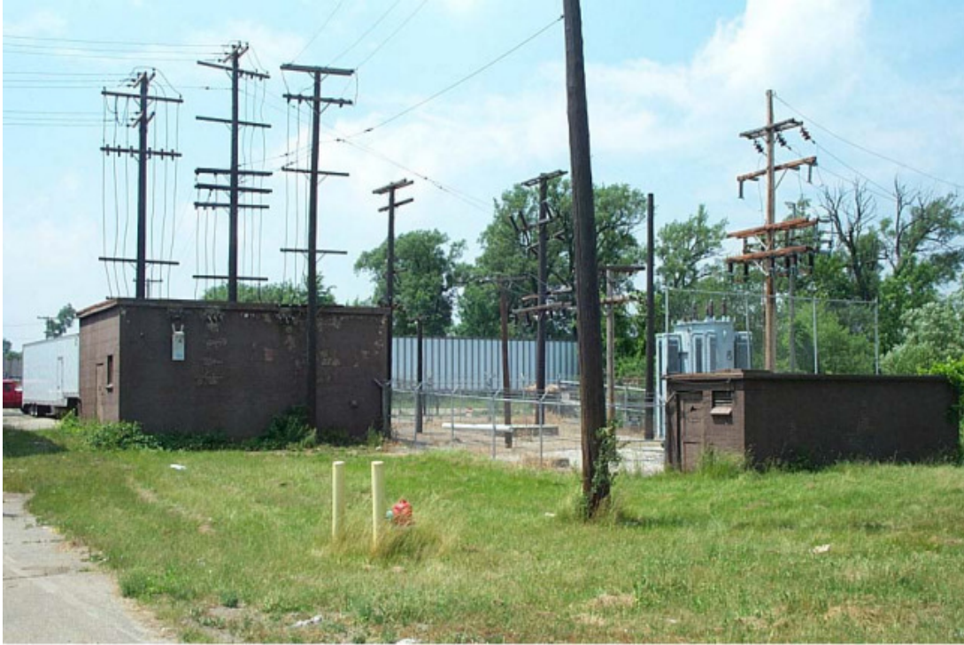
Photo 8. Utility structures I (left) & J, looking northwest. Photo by Burke Jenkins, Hamilton Anderson Associates, May 2002.
