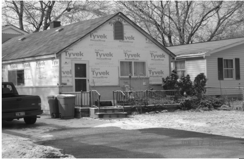
INCOMPLETE WORK ON STRUCTURES
