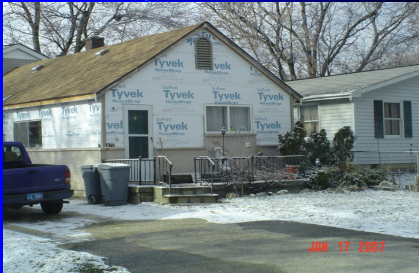
INCOMPLETE WORK ON STRUCTURES
