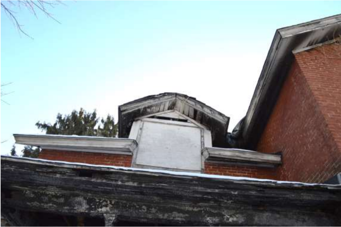
16 – North dormer showing fire damage, January 2021
