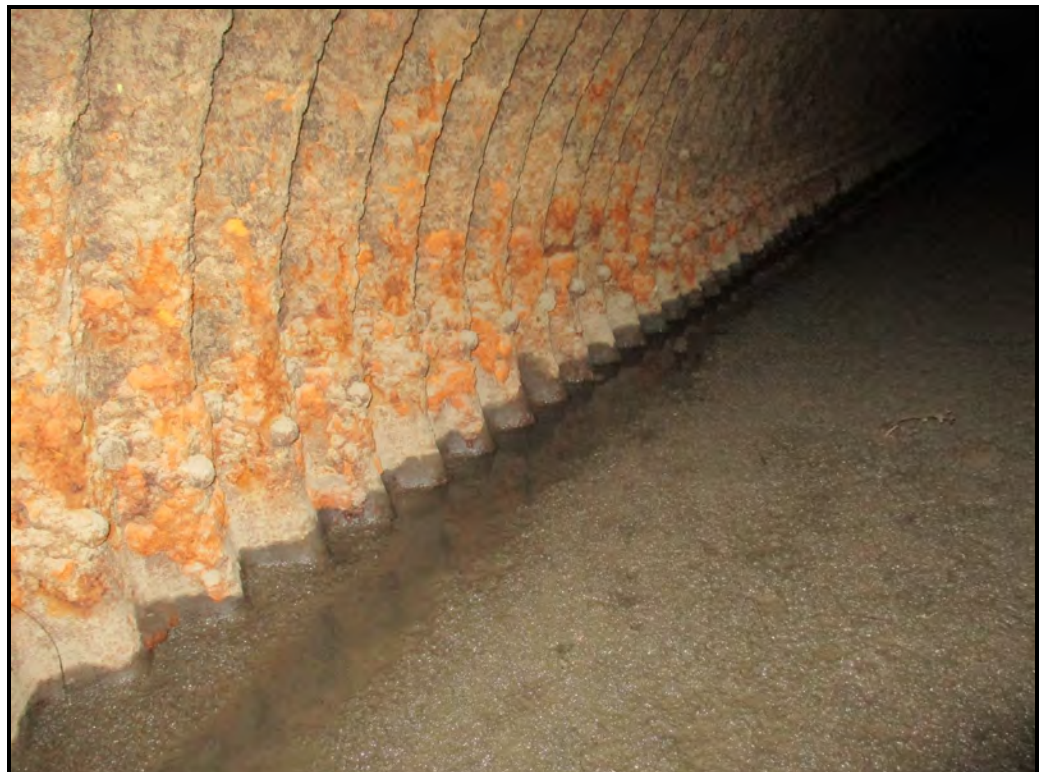
Rust and scale on CMP
