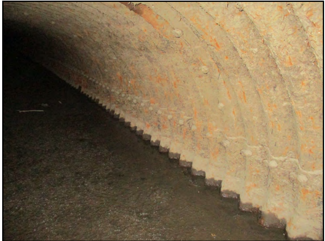
Rust and scale on CMP
