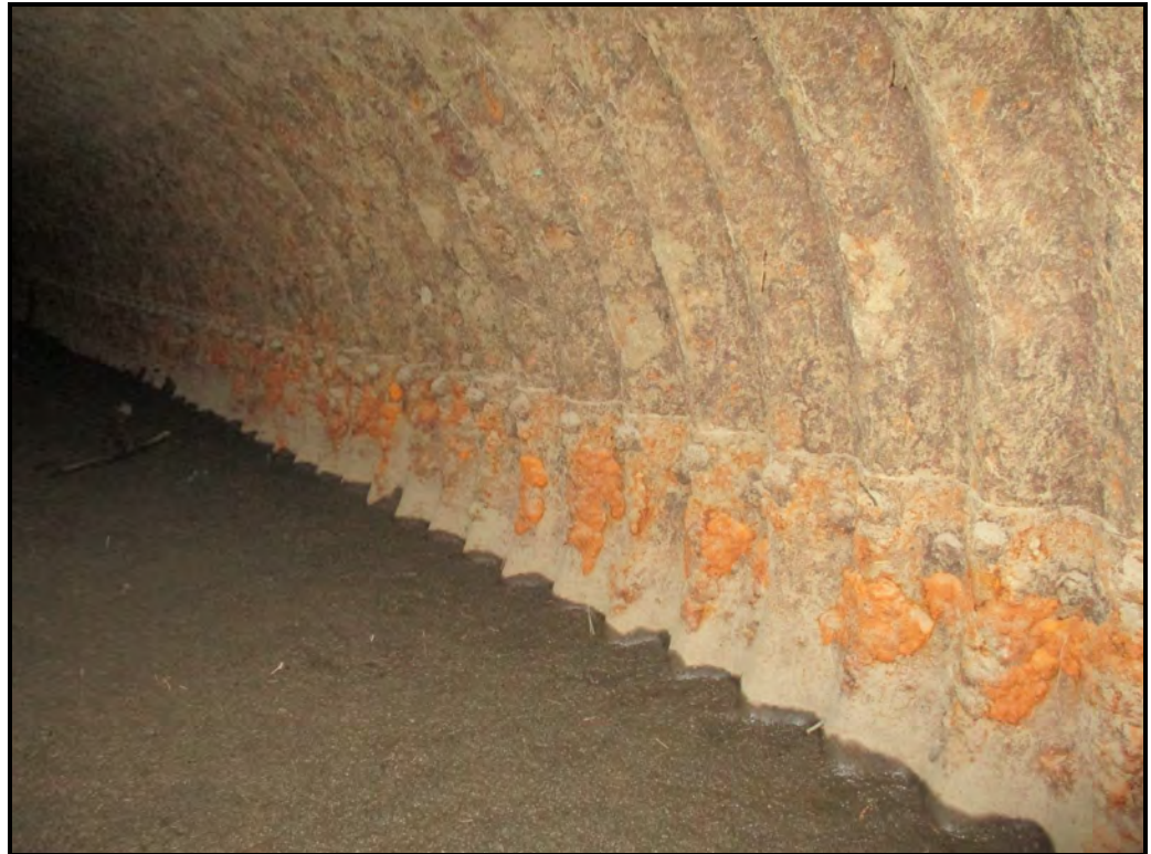
Heavy rust and scale on CMP
