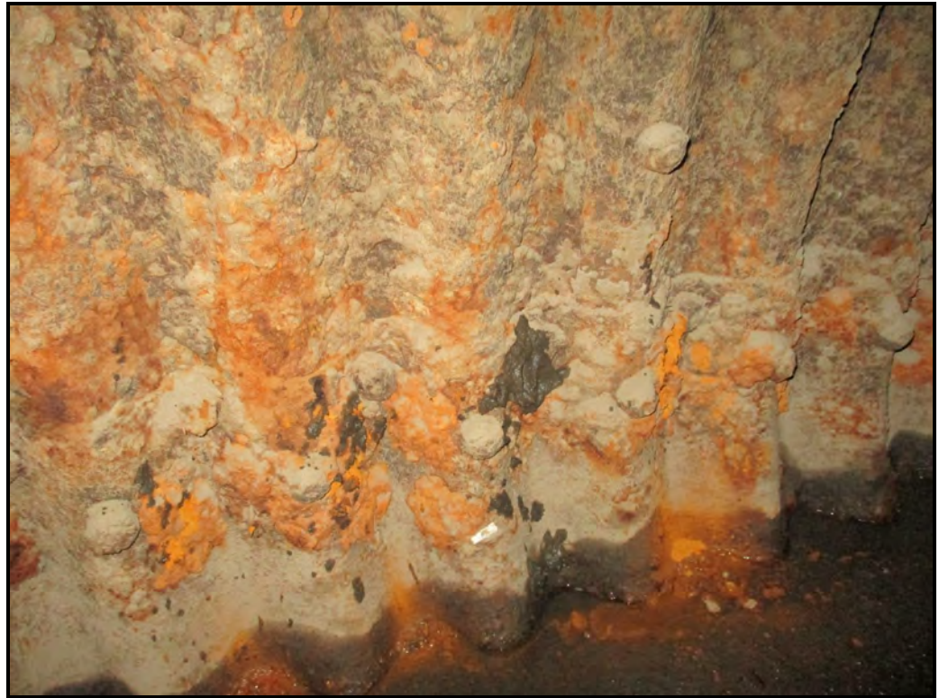
Heavy rust and scale on CMP
