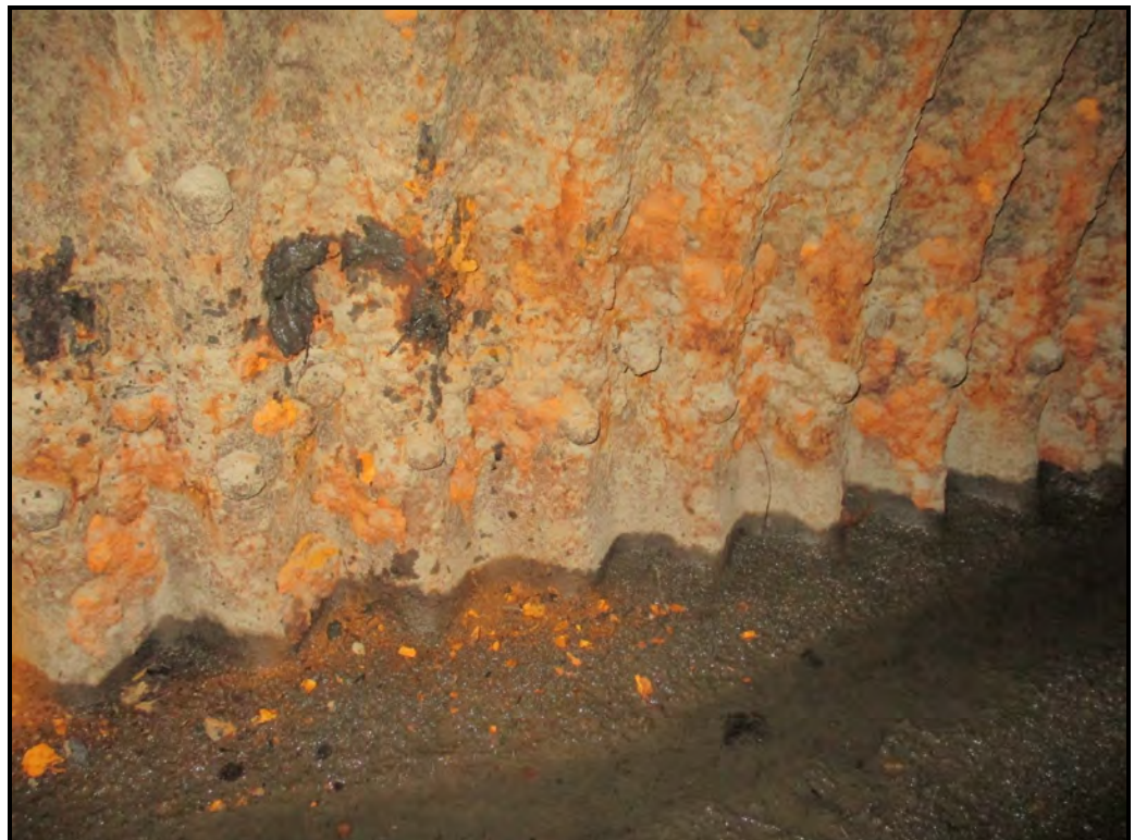
Heavy rust and scale on CMP
