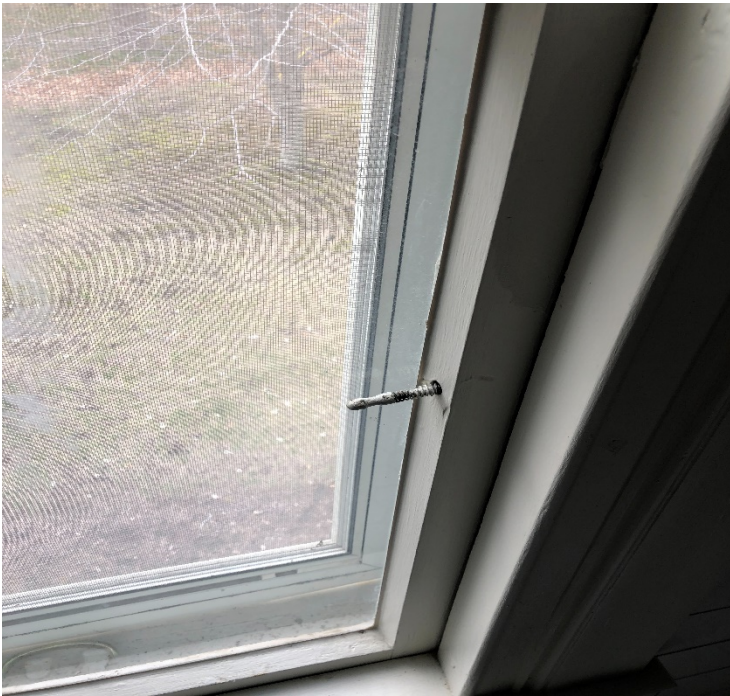
Windows rattle due to proximity to Dutton Road.
