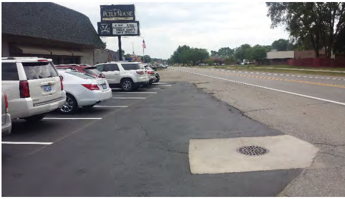
Looking east on the north leg of the intersection of Harrison and Auburn
