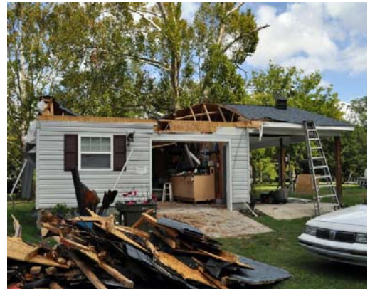
Wind Damage to a House
