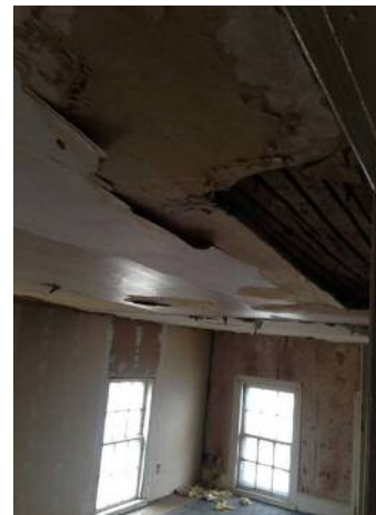
Water damage at ceiling from roof leaks.
