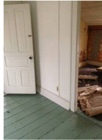
Water damage at walls and sags at floor with water damage.
