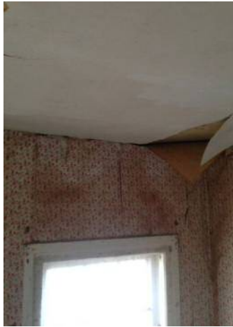
Water damage at ceiling.
