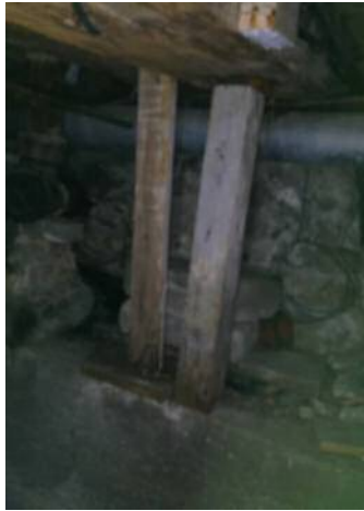
Improper support posts at crawlspace.
