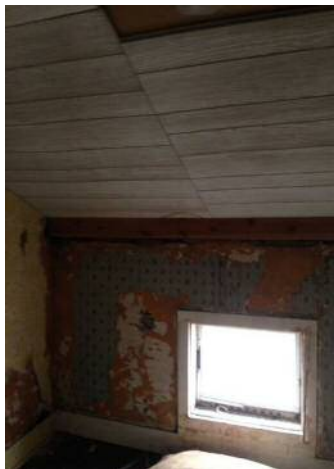
Water damage at ceiling and walls.
