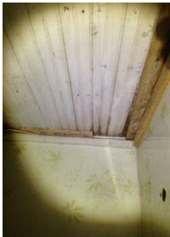
Water damage at lower level bathroom.
