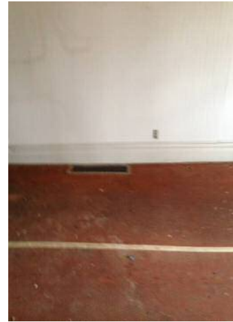
Water damage at subfloor, at wall, and sag at floor.
