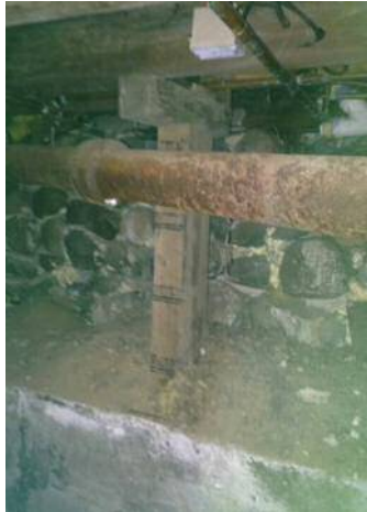
Corroded waste stack requires immediate replacement due to risk for sewage leaks.
