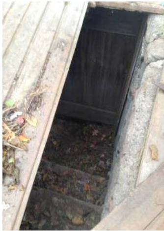
Damaged entry door down to walkout and rot observed at basement doors.
