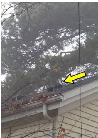
Damaged vent stack.
