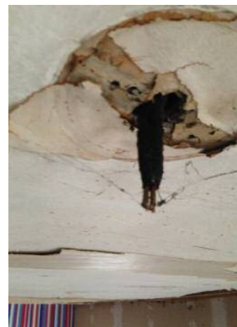
Exposed wires at ceiling, possible aluminum wires.
