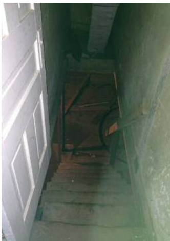
Basement stairs no longer level or structurally sound.
