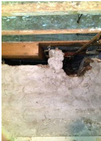
Damaged bearing wall, structurally unsound, and lean at load bearing wall.
