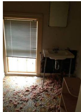
Water damage at second story bathroom.
