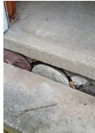
Loose field stone at porch and at rear structure.
