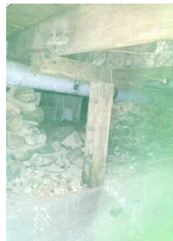
Improper support post at crawlspace.
