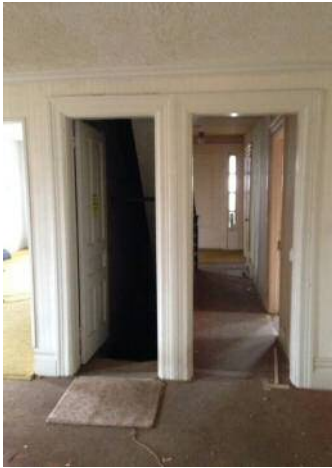
Sag at floor and at ceiling.
