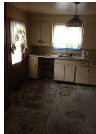
Water damage, mold growth, peeling paint, sagged floors.
