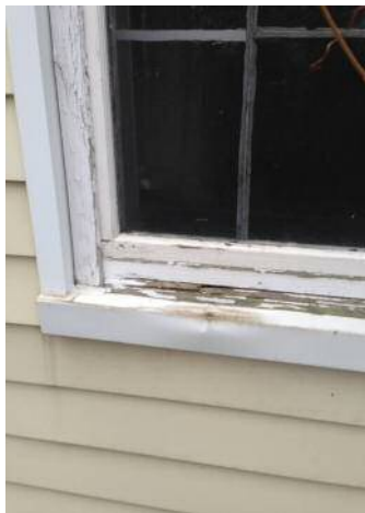
Peeling paint and rot at windows.
