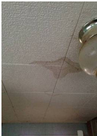
Water damage ceiling tile at rear addition. Possible asbestos tiles.
