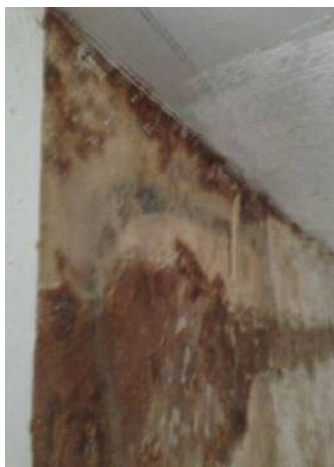
Heavy water damage at second story at rear of home. Mold growth observed.
