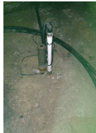
Pump at floor, provides evidence that basement floods.
