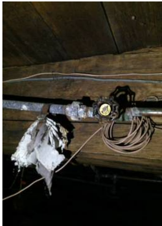
Pump at floor suggests basement floods.
