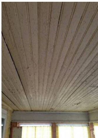
Peeling paint throughout home and risks to exposure to lead.
