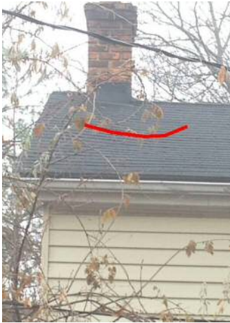
Observed sag at rear roof structure.
