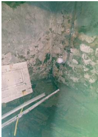
Water penetration and cracks at stone foundation wall.
