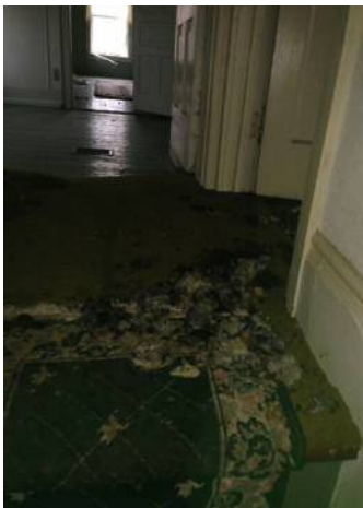
Water damage at second floor hallway and rodent excrement.
